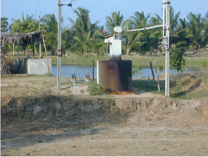
Pond protection—possible PCB contamination during runoff.
